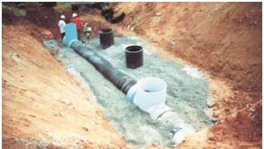
Backfill over the Water Quality Unit and installation of bypass line complete
